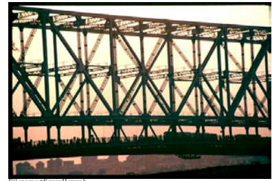
Figure 5.6: The Howrah bridge. Trusses are such a good idea that they are used recursively. The bars in some large trusses, like this one or the Eiffel Tower, are themselves made of trusses (courtesy Bipin Chandra, www.bipinchandra.co.uk ).
