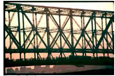
Figure 6.6: The Howrah bridge. Trusses are such a good idea that they are used recursively. The bars in some large trusses, like this one or the Eiffel Tower, are themselves made of trusses (courtesy Bipin Chandra, www.bipinchandra.co.uk ).
